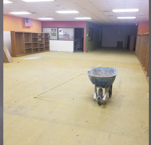
Flooring is being replaced in much of the school (Media Center pictured) as well as lockers.
