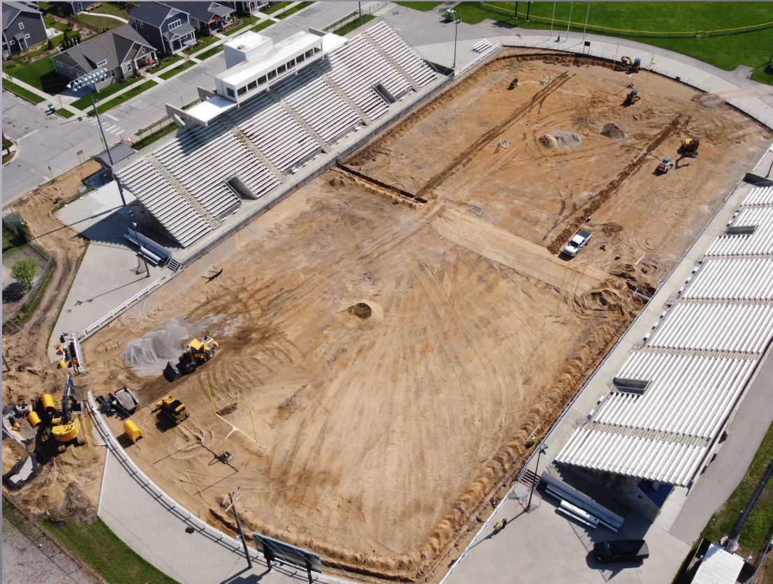
Existing synthetic turf is gone and preparations are underway for installation of the new turf.
