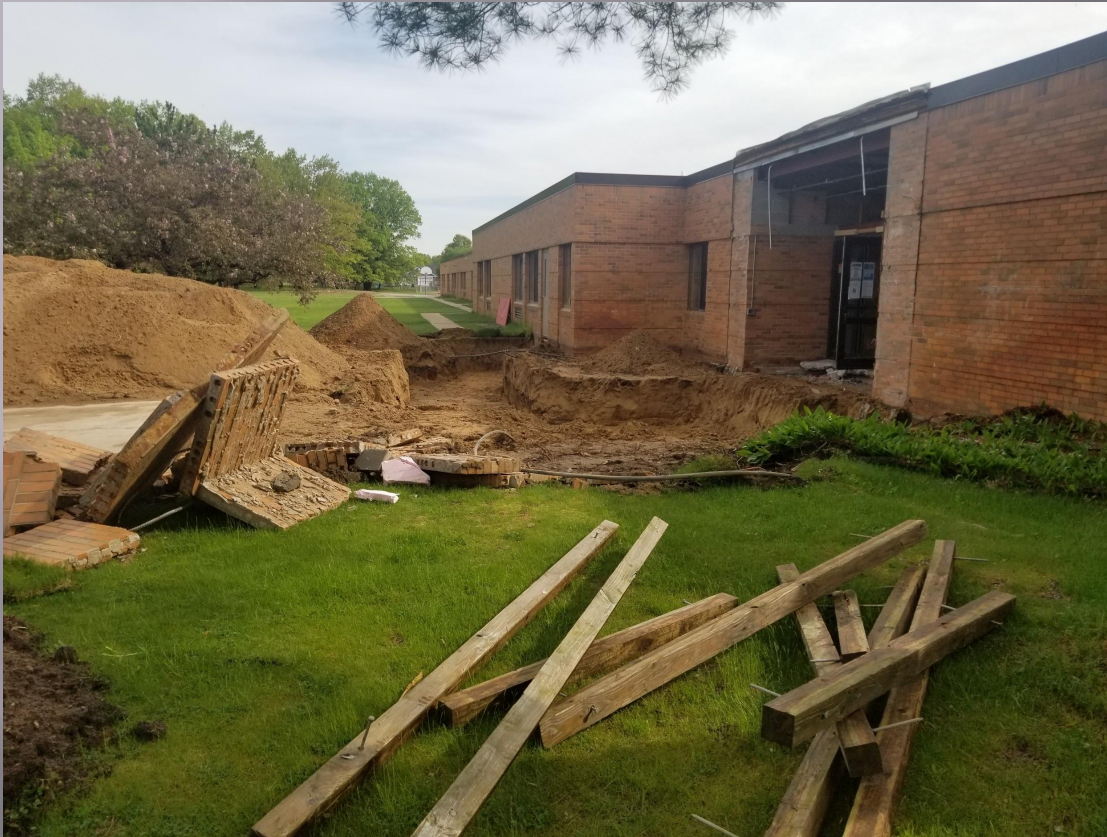
The front / main entry canopy has been removed. Prep work is underway for footings and foundations.
