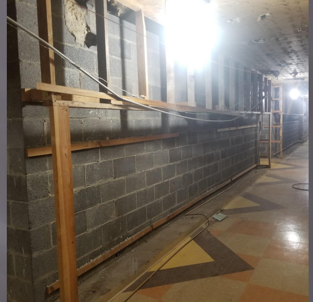
Phase II at Willow Hill includes four classroom renovations, Media Center upgrades, restroom renovations, mechanical and electrical systems upgrades, locker replacement and corridor upgrades.
