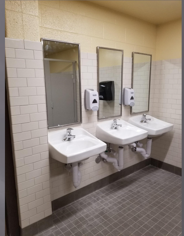
Restrooms need doors and final cleaning.
